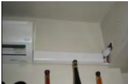
Indoor units located below window and too close to ceiling Source: Best Practices Installation Webinar, NEEA
