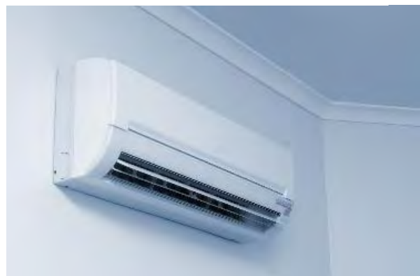
Exhibit 27: Properly Installed Ductless Indoor Unit
