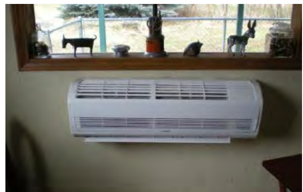
Exhibit 22: Bad Location for Ductless Indoor Unit
