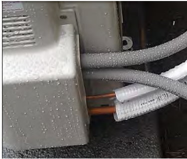
Line set not properly insulated Source: Best Practices Installation Webinar, NEEA
