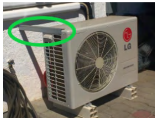
The outdoor unit attached at the top to prevent it from falling over
