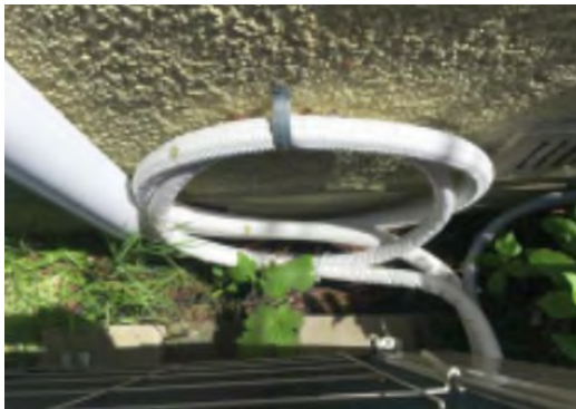
Excess line set not removed but coiled up
