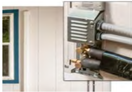
Line set properly insulated Source: Best Practices Installation Webinar, NEEA
