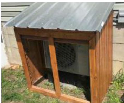
Decorative shed over outdoor unit with very little air space to the house wall
